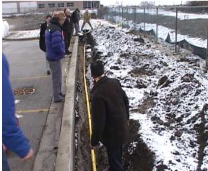
Figure 18: PA12 Flow Loop Installation
