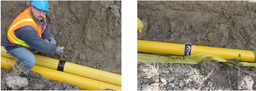
Figure 17: Illustration of the installation and leak testing of a 6x2” Continental Industries mechanical fitting. The mechanical fittings were installed at 250 psig and tapped with no observed issues.
