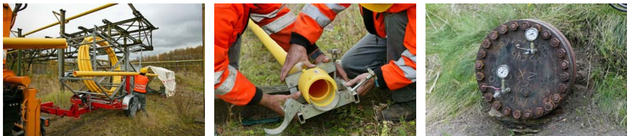
Figure 18: illustrations of Ruhrgas installation operating at 345 psig
