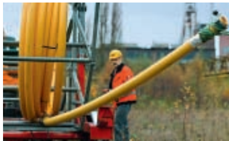
Until now, gas pipes have been made of steel; today engineers can lay flexible VESTAMID pipes that are no less sturdy
